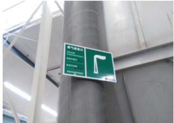
干坯切割机除尘器排气筒 P14
