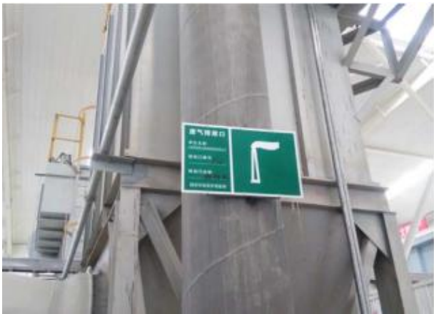
干坯切割机除尘器排气筒 P15
