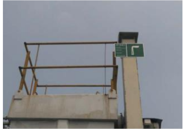
粉煤灰料仓除尘器排气筒 P 4
